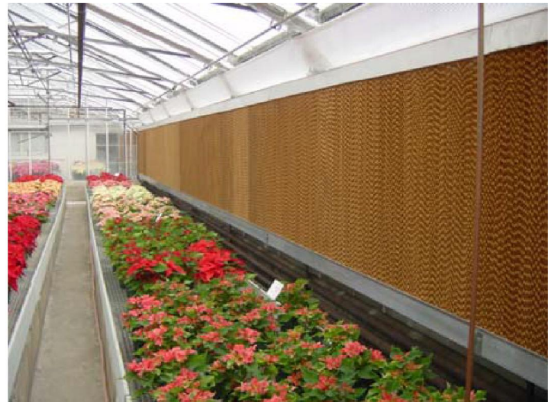
Evaporative cooling pad installed along the inside of the ventilation inlet opening.
